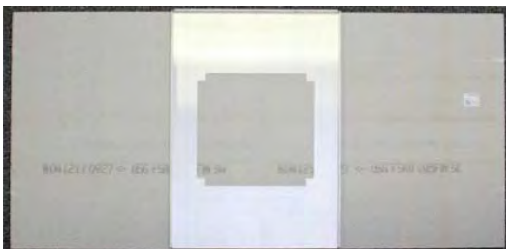
Figure 4: Ceiling Tile Brace on ceiling tile
